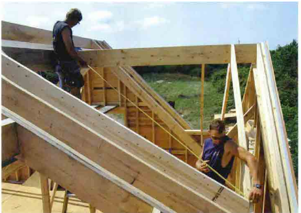
Measuring an irregular valley. The quickest way to figure out the irregular valley is to stretch a line from corner to corner. Here, a measurement is taken along that line.
