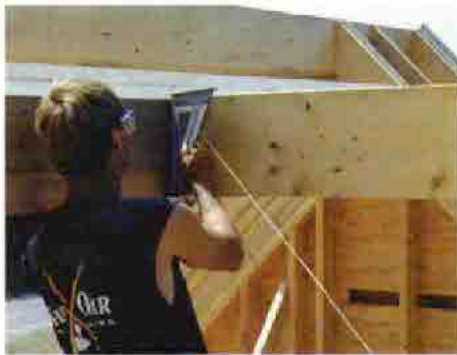
Finding the plumb cut. A rafter square held in the corner against the string determines the angle of the valley plumb cuts.
