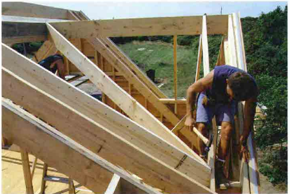
Valley rafter slips into place. After all the angles have been cut into the valley rafters, including a bevel on the bottom edge where the ceiling planes intersect, the valleys are nailed in permanently.
